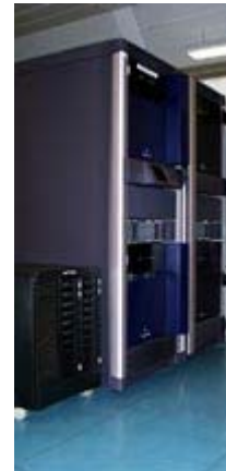
Figure 1.10 Supercomputer at VR•C
